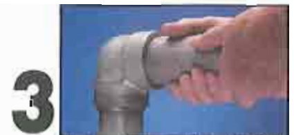
3 Fitter inserts pipe into fitting. Gap-A-Let® ring automatically assures the required minimum gap (1/16") to meet the code requirements of ANSI 31.1 Section III, ASME & military codes.
