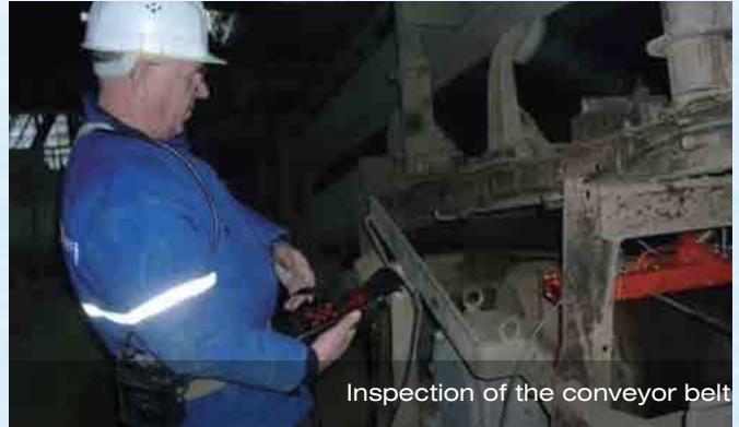
Installation of the scanner above the belt at driving drum of conveyor
